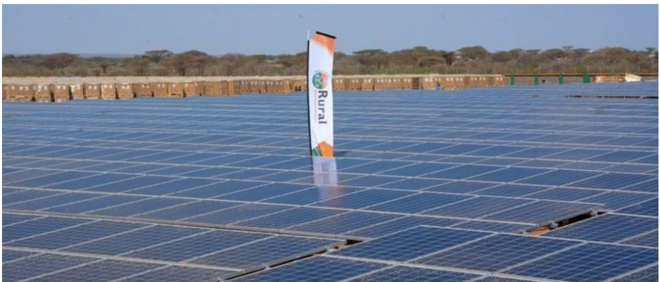
Figure 3: Garissa Solar Photovoltaic Power Plant
