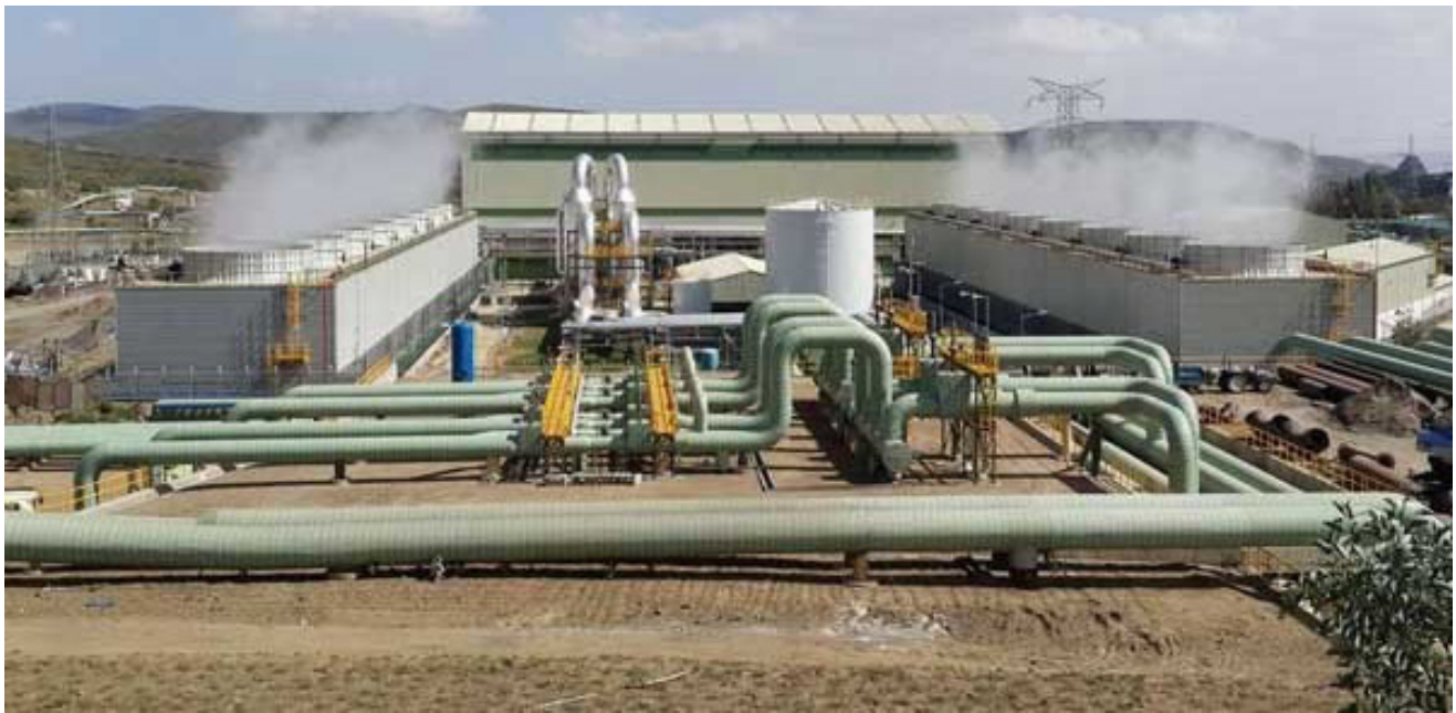
Figure 2: Olkaria 280 MW Geothermal Plant
