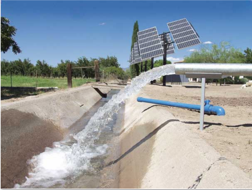
Water pumping using solar energy
